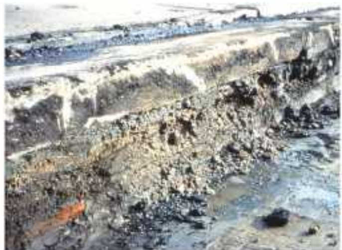
b) Aggregate contamination or degeneration
