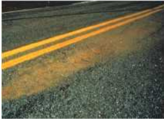
c) Subgrade pumping
