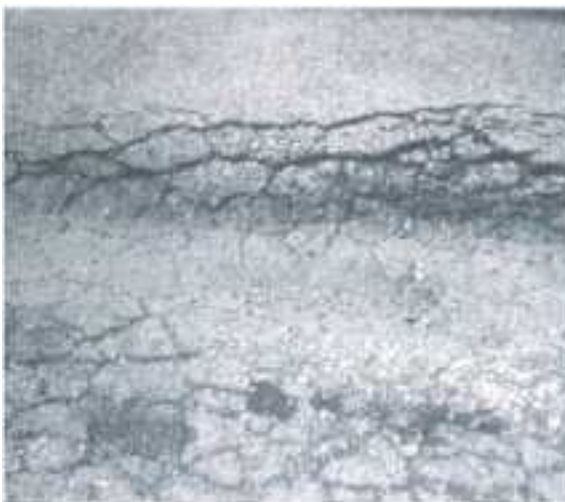
a) Excessive rutting
